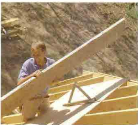
Staging goes on before the courses go up. After the first course of sheathing is nailed off, roof brackets are nailed in and planks are set before the next course is started. Staging provides a safe place to stand as well as a place to rest the sheets for the next course.
