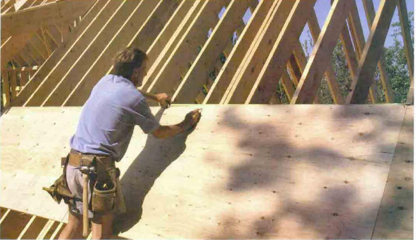
The sheathing straightens the rafters. Before nailing off the sheathing, a tape is hooked to the rafter on one end, and the rafter layout is marked along one edge. The rafters are then moved to the mark and nailed in place.
